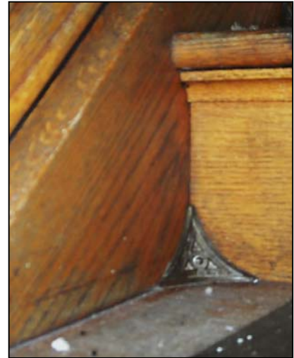
Figure 3.8. Triangular, cast iron members were installed in the corners created in the staircase to prevent dust buildup. Photo courtesy of author.
