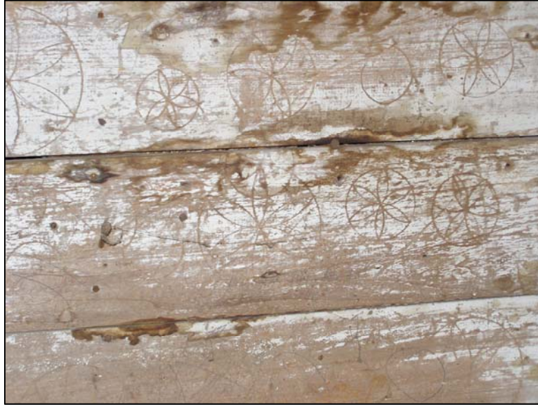
Figure 6.34. Hexafoil symbols on an interior plank wall of a grist mill near Staunton, Virginia. Photo courtesy of Thomas Cundiff.
