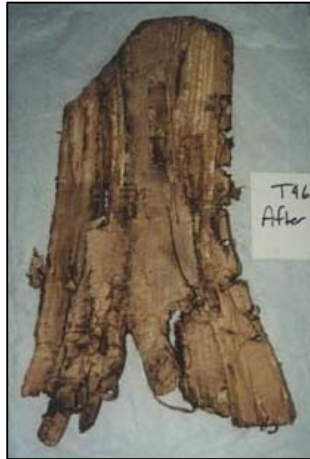
Figure 6.6. Stays found in the attic or roof of the Hammond-Harwood House, Annapolis, Maryland. Photo courtesy of the Hammond-Harwood House Association (Titman 2011b).
