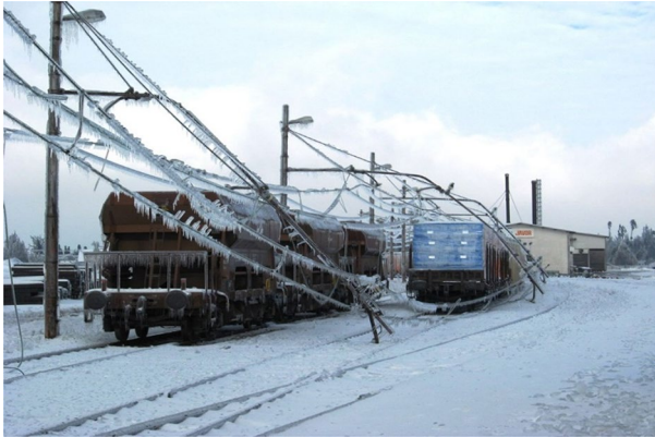
Fig.1 Overhead lines damage due to ice accretion (The Railway Transport Union of Slovenia 2014)
