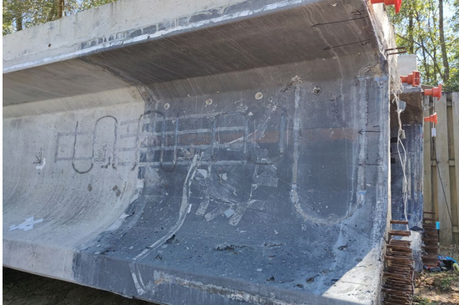
Figure 234: The result of scanning a bridge member (G6E1) containing self-compacting concrete (SCC) with no fibers, and UHPC with fibers. The top figure shows the bridge member G6E1 with the darker portions (end portion) as the UHPC and the lighter portion (remaining portion) as the SCC without fibers
