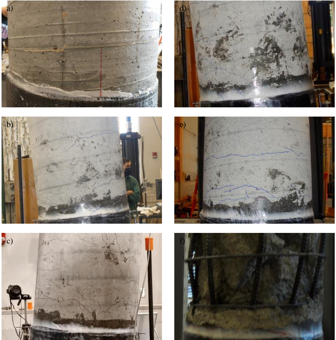
Figure 3.23. Concrete Damage Above Jacket at 20\delta/\delta_y (at 15\delta/\delta_y for C(CFRP)-4.0-#7(1.3)-0.15) for: a) C(CFRP)-4.0-#7(1.3)-0.05, b) C(CFRP)-4.0-#5(1.4)-0.05, c) C(CFRP)-4.0-#7(2.7)-0.05, d) C(CFRP)-4.0-#7(1.3)-0.05-EQ, e) C(CFRP)-4.0-#7(1.3)-0.05-2X, and f) C(CFRP)-4.0-#7(1.3)-0.15
