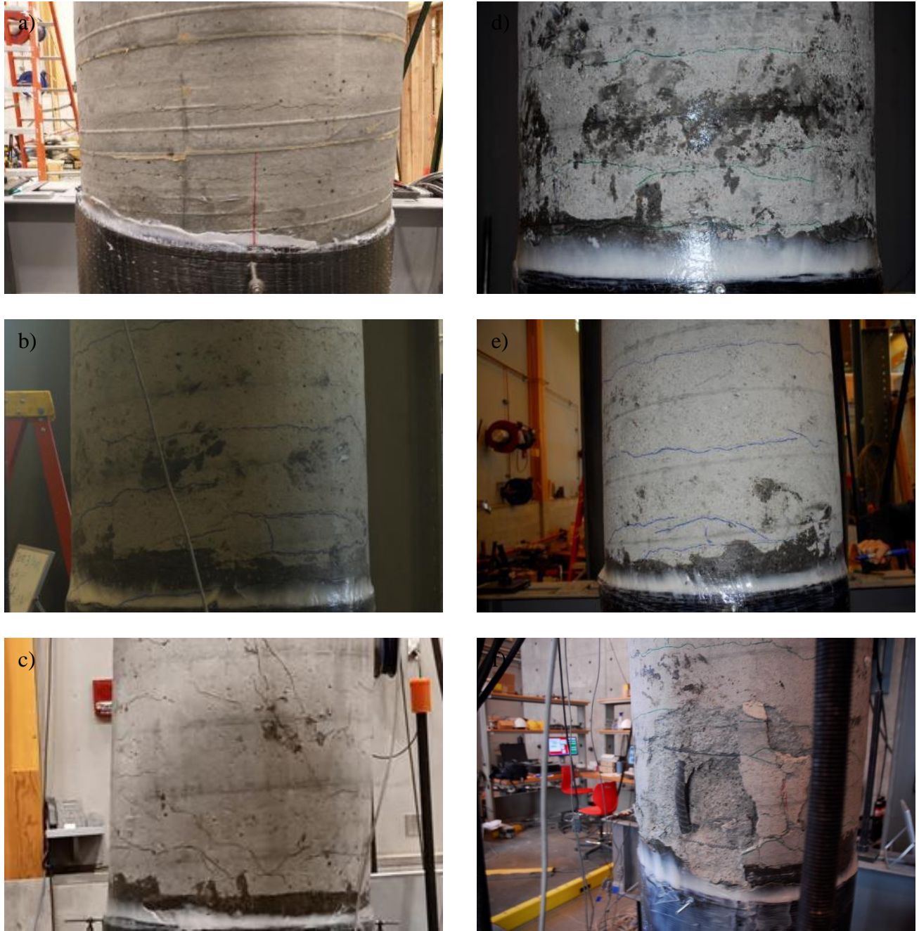
Figure 3.21. Concrete Damage Above Jacket at 15\delta/\delta_y for: a) C(CFRP)-4.0-#7(1.3)-0.05, b) C(CFRP)-4.0-#5(1.4)-0.05, c) C(CFRP)-4.0-#7(2.7)-0.05, d) C(CFRP)-4.0-#7(1.3)-0.05-EQ, e) C(CFRP)-4.0-#7(1.3)-0.05-2X, and f) C(CFRP)-4.0-#7(1.3)-0.15
