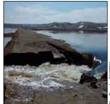
Climate change will impact roads on FWS managed lands. Road damage due to flooding at Arrowwood NWR (top); washed out bridge at Flint Hills NWR (bottom).
