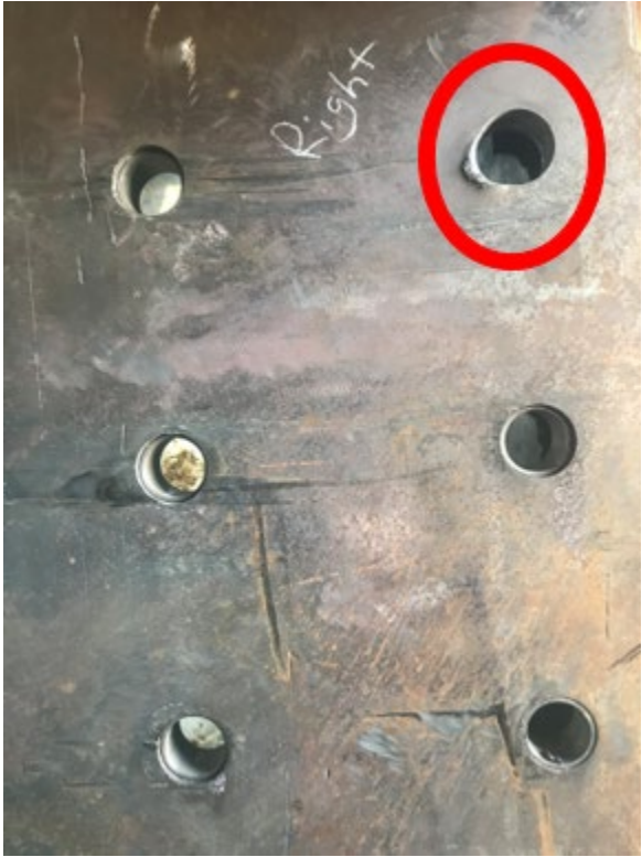
Figure 76. Draft pocket deformed bolt hole
