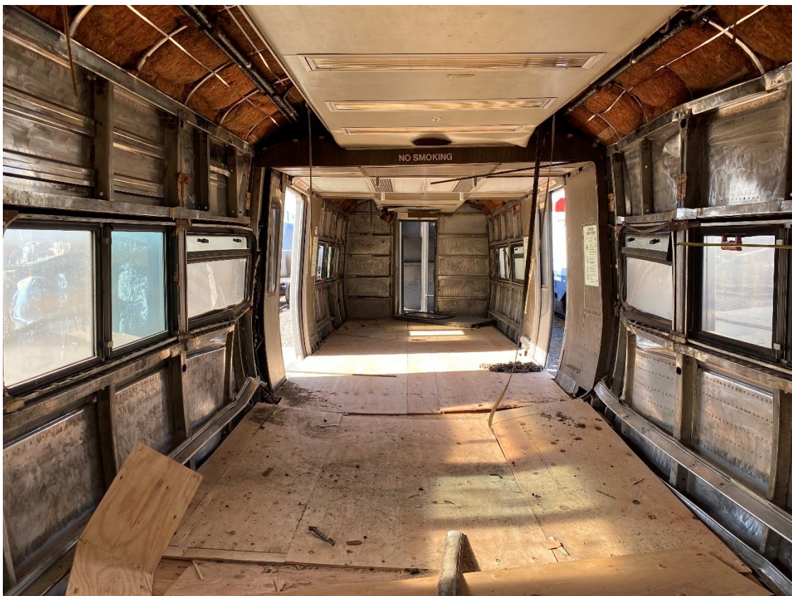
Figure 83. M1 interior damage, buckle at rear door
