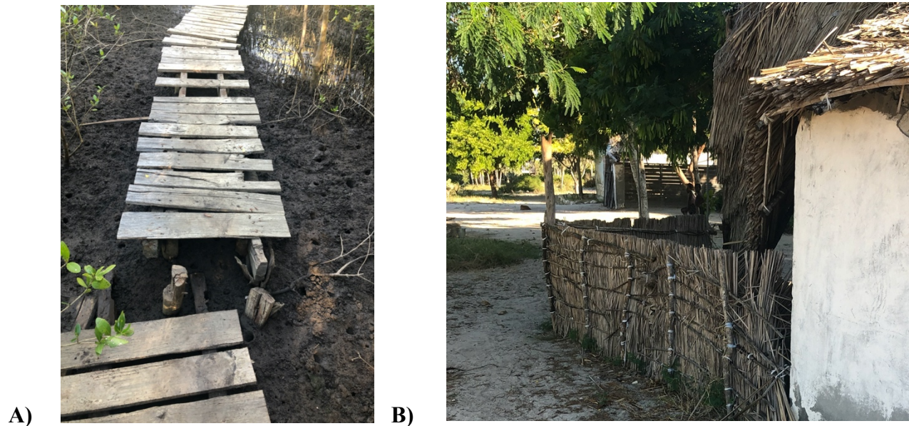
Figure 11. A) A part of the boardwalk in need of maintenance. B) A structure damaged by the recent cyclone Freddy.
