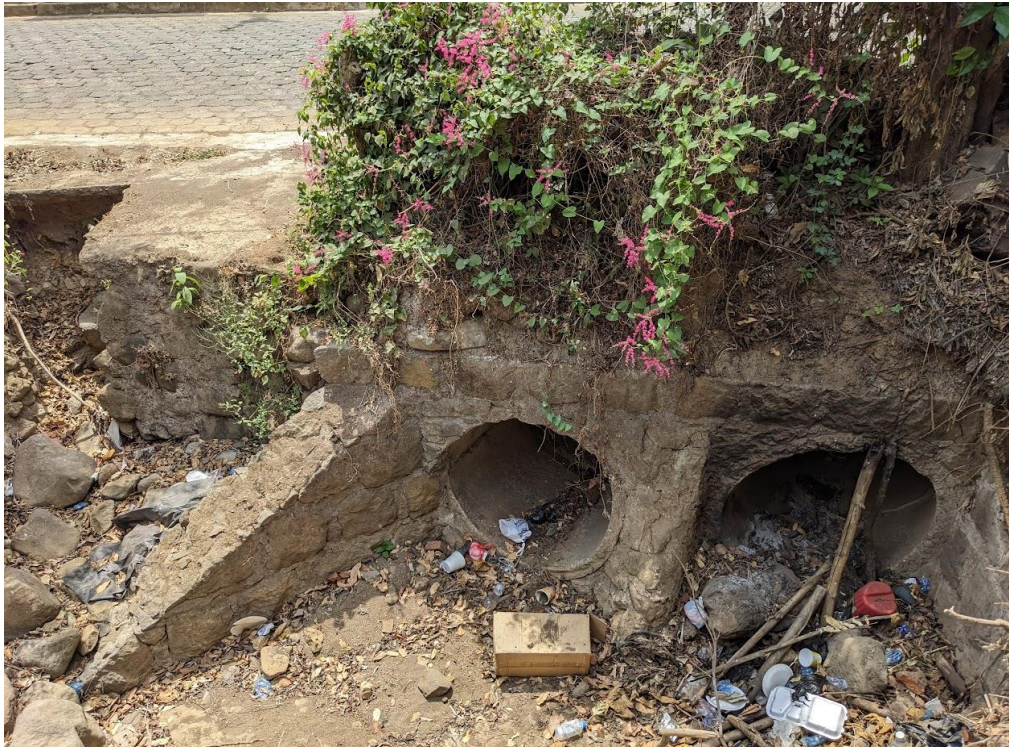
Figure 14: Culvert at the end of the La Claros drainage where water overflows and floods the road above.
