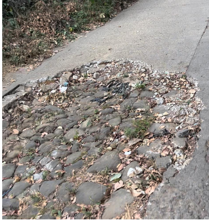
Figure 11: Old Road damage caused by past flash flood events.
