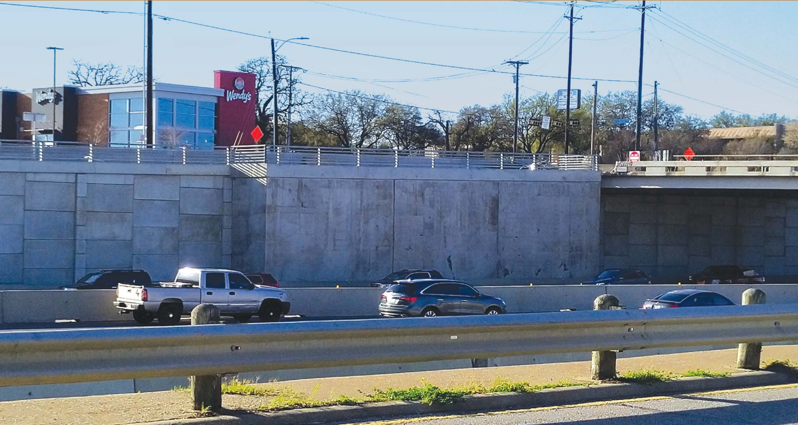
Highlighting the revised design (extended portion) of the retaining wall on TX 360 north of IH 30. This portion of the retaining wall was extended due to a change in the foundation design to mitigate a conflict with a utility duct bank.
