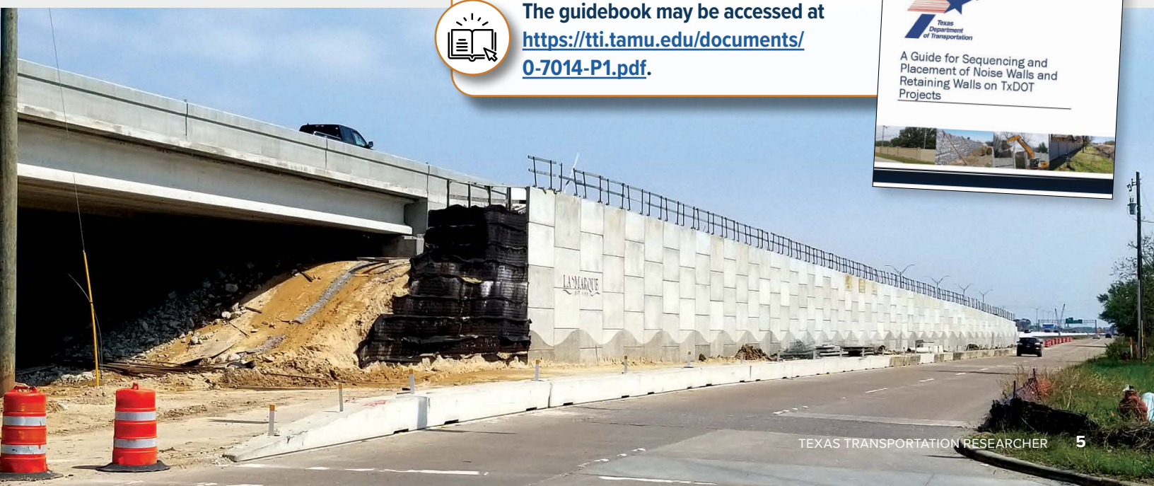
Retaining wall widening to facilitate the addition of main lanes on IH 45 near FM 1765 in the Houston District.
