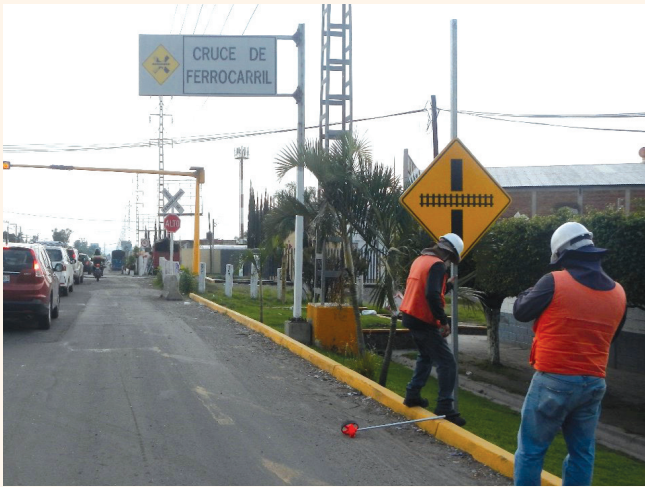
Road workers by the Zapopan Air Force Base install a railway crossing intersection sign.
