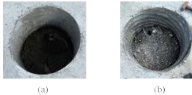
Figure 3-52: Surface finish after removal of pipe with (a) sonotube and (b) corrugated pipe.
