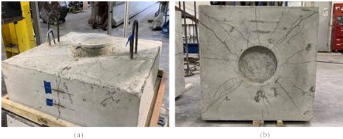
Figure A - 53: Cracking on (a) cap and (b) bottom of the Specimen S2-6
