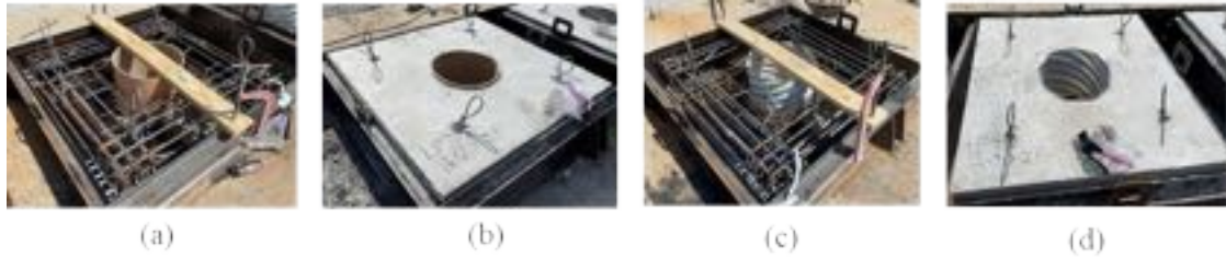
Figure 3-51: Construction and casting of cap: (a) placement of reinforcement and (b) casting of cap concrete for specimen with Sonotube and (c) placement of reinforcement and (d) casting of cap concrete for specimen with corrugated metal pipe.
