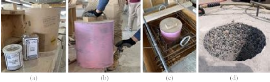
Figure 3-7: Procedure for achieving exposed aggregate finish: (a) application of polyurethane clear coat, (b) application of set retarding agent, (c) placement of void in cap, and (d) finish after pressure washing surface
