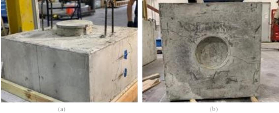
Figure A - 23: Cracking on the (a) east side and (b) bottom of specimen S2-1
