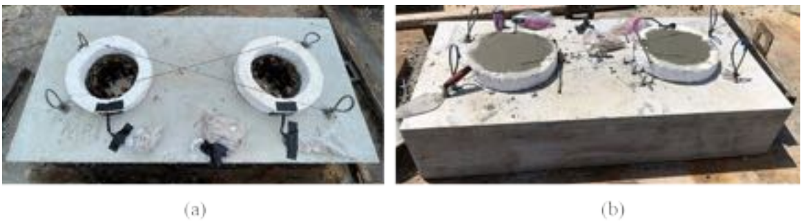
Figure 3-62: Casting of the plug: (a) 3-inch form and reinforcement was placed and (b) concrete was cast.
