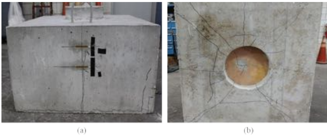
Figure A - 106: cracking on the (a) east side and (b) bottom of specimen S2-16
