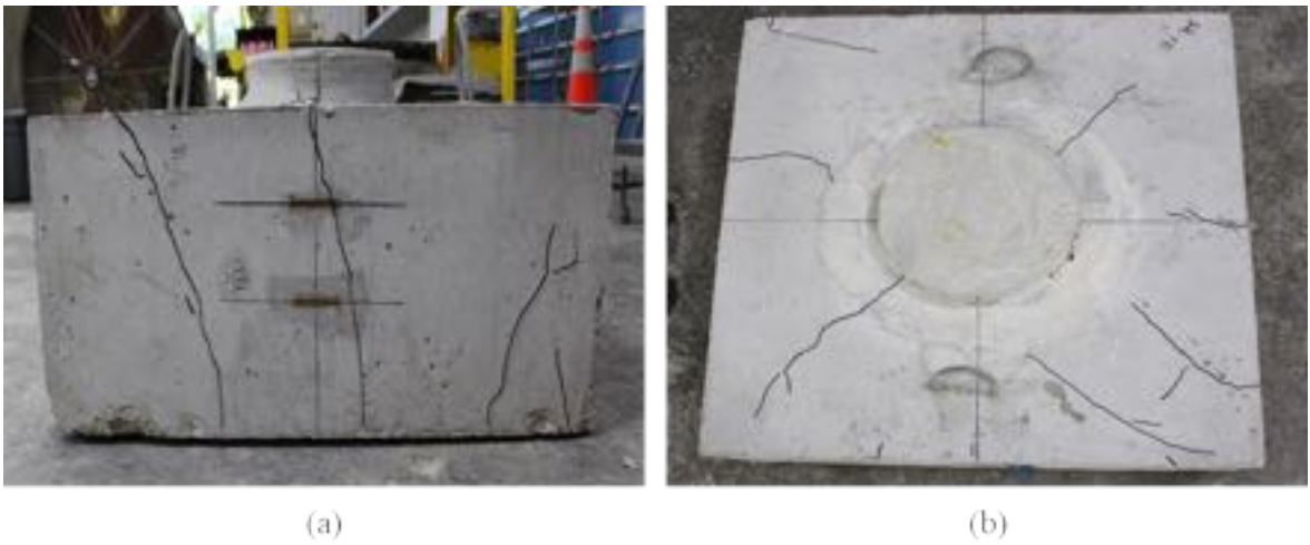
Figure A - 103: Cracking on the (a) north side and (b) top of the cap
