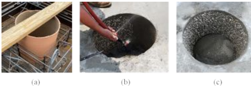
Figure 3-56: Exposed aggregate finish: (a) pipe with the set retarding agent, (b) pressure washing the surface, and (c) surface finish.
