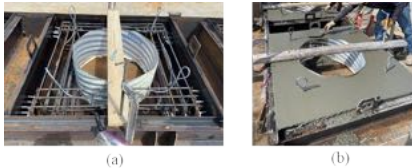
Figure 3-68: (a) construction of the socket connection specimen and (b) casting of the cap.
