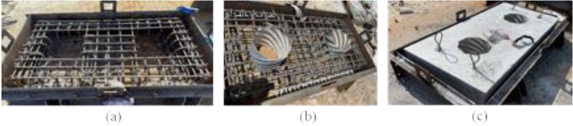
Figure 3-61: Construction and casting of multi-plug specimens: (a) reinforcement layout, (b) corrugated pipes placed, and (c) after concrete had hardened.
