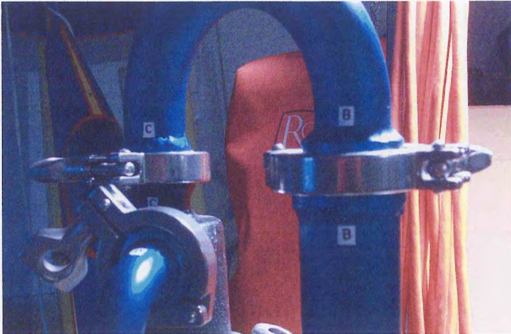
U-tube to control tube and cyclone to U-tube connection.
