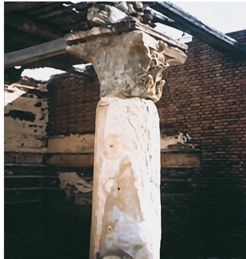
Figure 3B. Inside Omar Ibn Al-Aas Mosque, Damietta. Salt weathering of marble.
