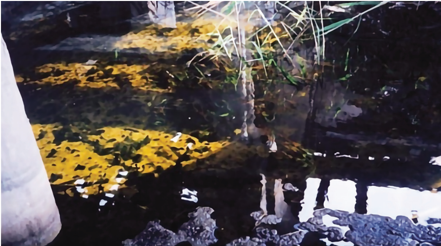
Figure 4. Bacterial colonies growing close to the marble columns of historical mosques; algae growth, and the spread of ground water inside the courtyard of Omar ibn Al-Aas Mosque, Damietta.
