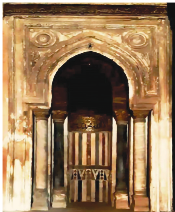
Figure 2A. Damaged marble of the archaeological Mihrab, Ahmed Ibn Tulun Mosque, in Cairo, Egypt.
