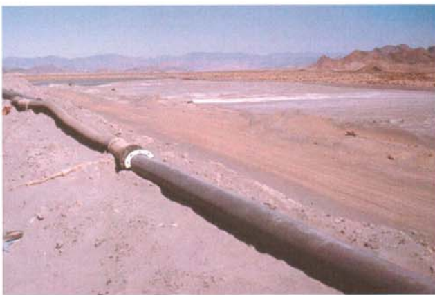
Flotation tailings slurry is discharged onto heap via a pipeline.
