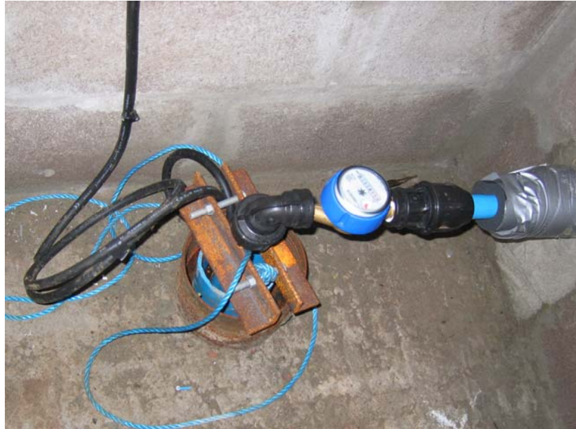
Figure 10 Typical well head construction of private boreholes in southern Scotland. The floor is cemented and the borehole open, but protected within a small shed.
