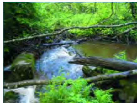
Dilapidated weir structure upstream from ALP-5.
