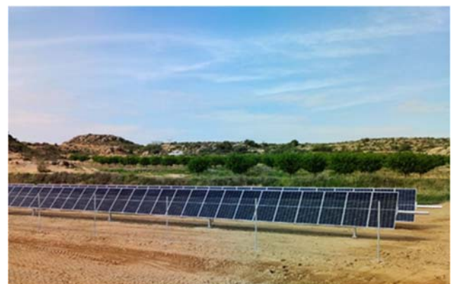
Fig. 1. Stand-alone solar photovoltaic water pumping installation for irrigation. Photovoltaic tracker on North-South axis. It allows us to follow the daily East-West path of the sun.
