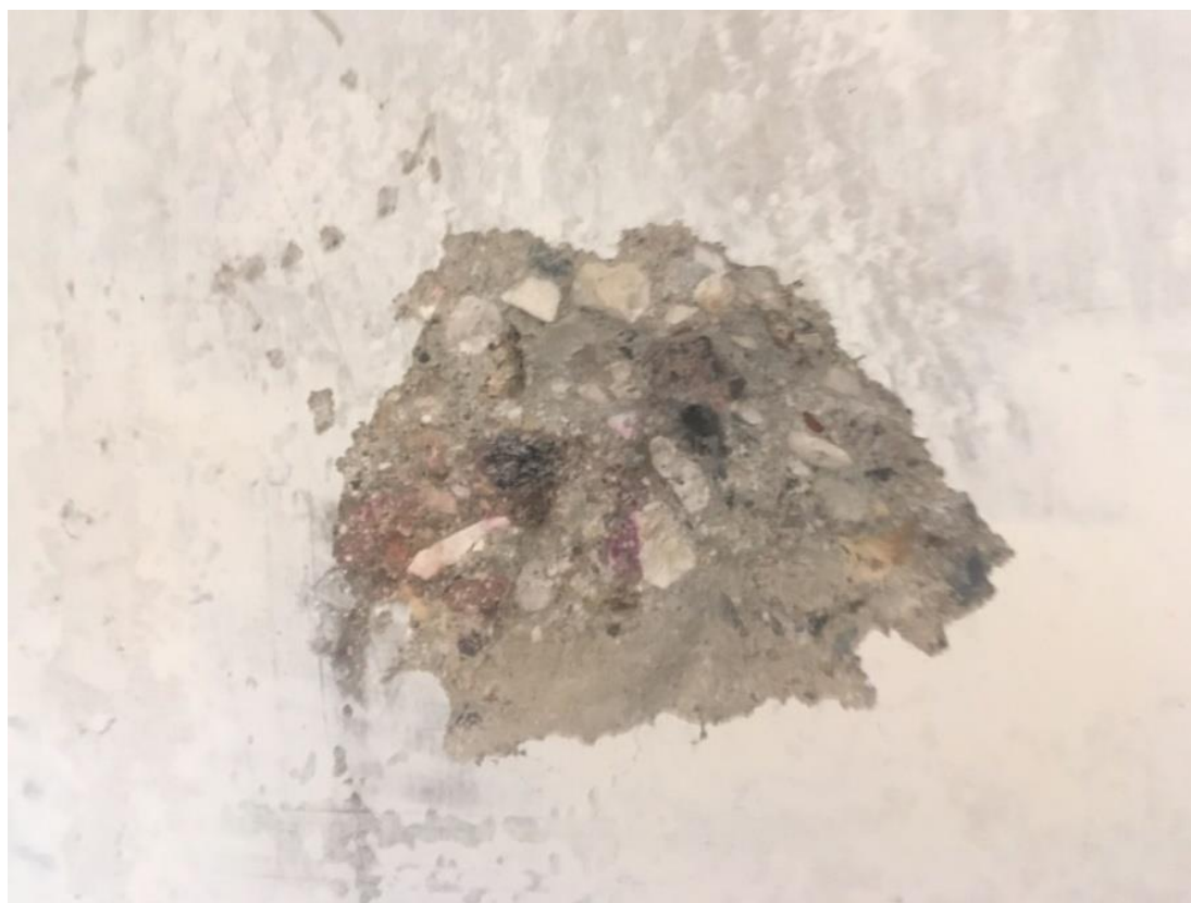
Figure 3. Absence of visible signs of concrete carbonization from the results of phenolphthalein test
