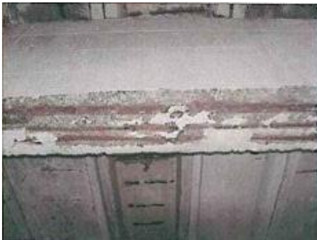
Figure 1. Corrosion of reinforcing bars in a beam
