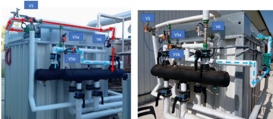
Fig. 2. Real view of the PCM-based TES system with connection pipes and valves
