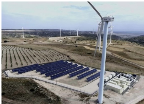
Fig. 4. La Plana hybrid facility
