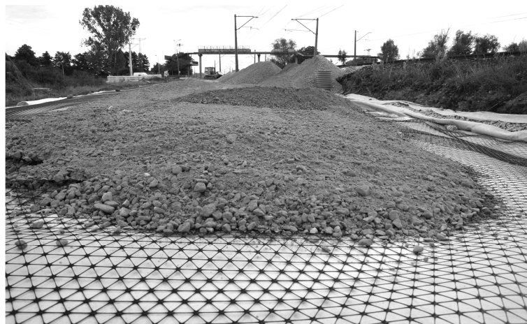
10. Laying the first layer of triaxial geogrid during the modernization of the E65 line in the area of LCS Gdańsk
