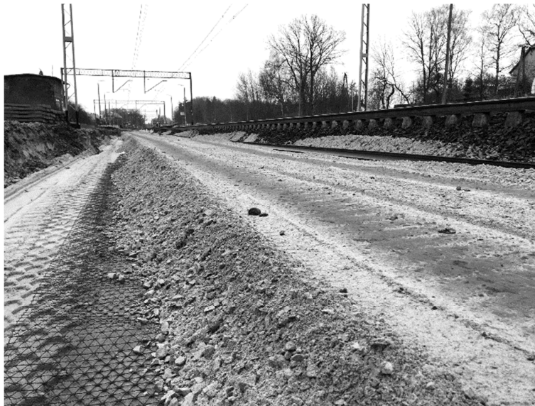
11. Stabilization of the protective layer during the modernization of the LK 273 line
