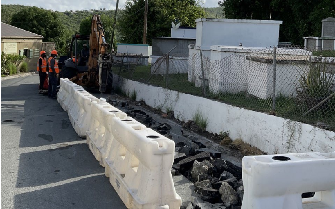
Figure 33. General view of the Upper Cemetery along with ongoing conduit excavation. View to northeast.
