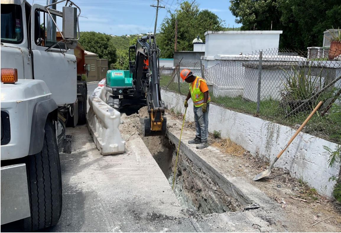
Figure 6. WAPA contractor, SSVI, and excavation of conduit trench near the Cruz Bay Public Cemetery. View to north-east.
