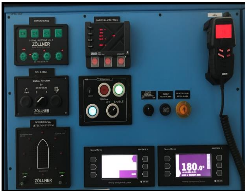
FIGURE 3-7: BRIDGE CONSOLE (SOURCE: OWN ELABORATION)
