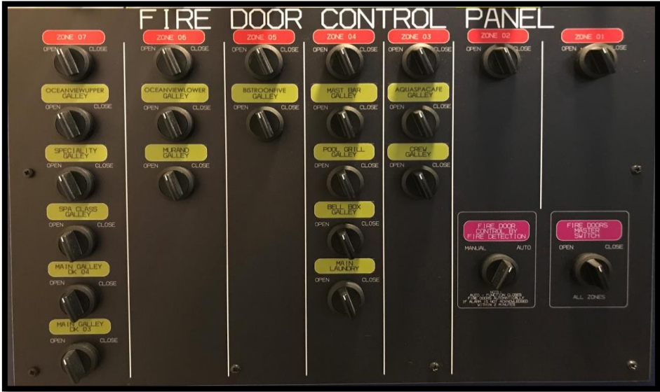
FIGURE 6-3: FIRE DOOR CONTROL PANEL (SOURCE: OWN ELABORATION)
