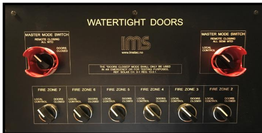
FIGURE 6-5: WATERTIGHT DOOR REMOTE CONTROL PANEL (SOURCE: OWN ELABORATION)
