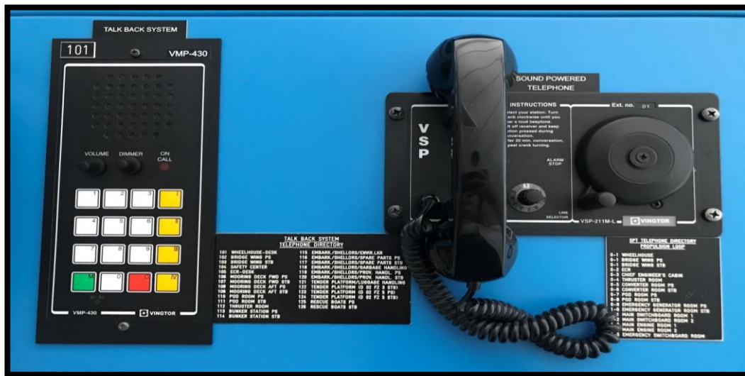
FIGURE 4-9: TALK BACK SYSTEM AND SOUNDED POWERED TELEPHONE WITH DIRECTORY (SOURCE: OWN ELABORATION)
