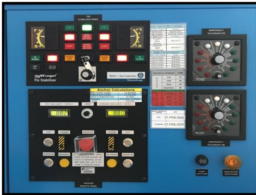
FIGURE 3-8: BRIDGE CONSOLE (SOURCE: OWN ELABORATION)
