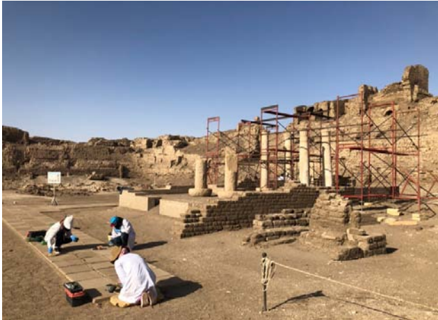
Figure 47: The conservators during the final restoration works of clay tiles of walkway.
