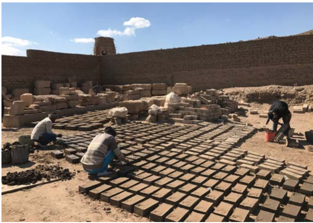
Figure 31: Workers add the mixture (clay & straw) to the mold for making adobe bricks.
