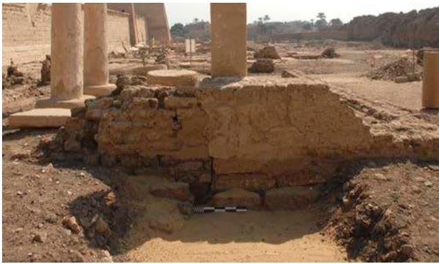
Figure 14: The state of conservation of the old mud brick foundation before the restoration works.
