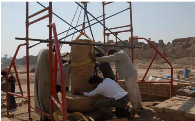
Figure 40: Senior conservator Lotfi, the Auther & assistants replace the shaft part of the column on original base of the southern side.
