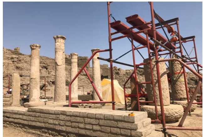
Figure 41: Shows the replacement of the two columns (with large parts missing) that were laid on the ground in final phase.
