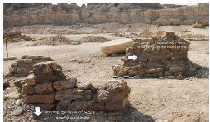
Figure 13: The state of conservation of the old mud brick walls before the restoration works.
