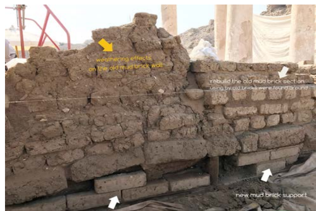
Figure 33: Shows the condition of the inclined wall in action to be restored & supported.
