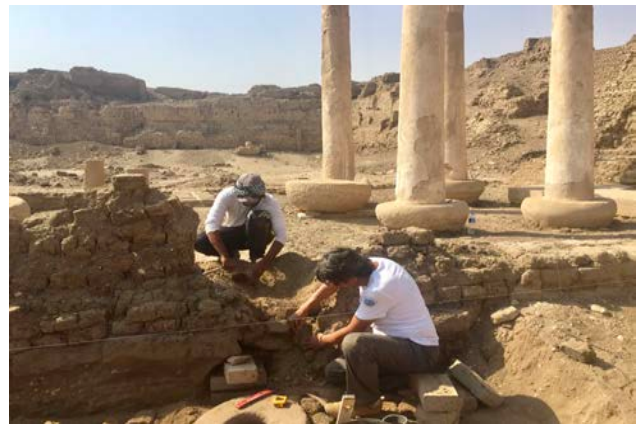
Figure 32: The senior conservator, Lotfi Hassan, the Author disassembles the inclined sections to clean, strength and rebuild them in the right position.
