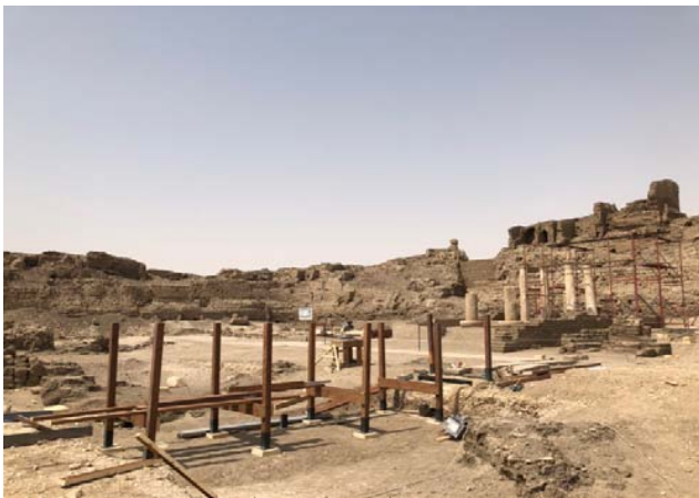
Figure 48: The construction of wooden bridge on archaeological features to protect it and to do way to reach the walkway to visit the butehamon house.
