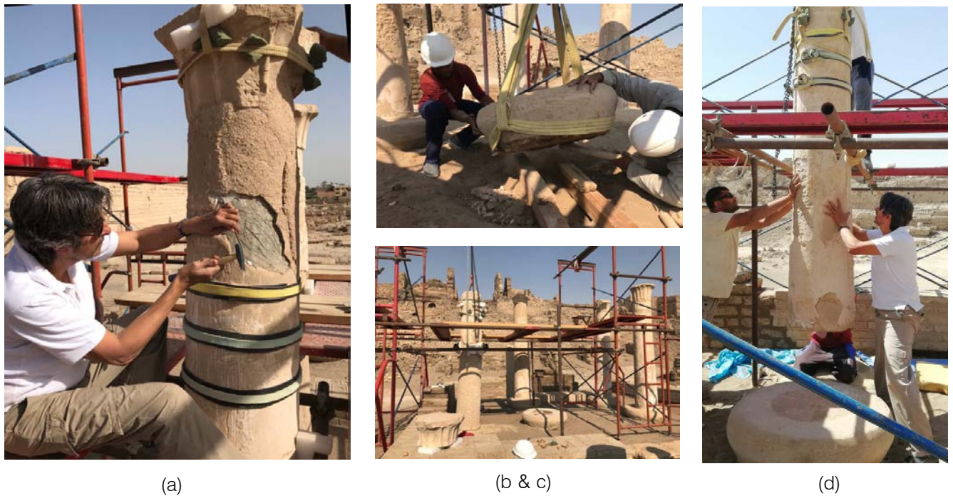
Figure 44: The author during removing the cement between the capital and the column shaft in preparation of dismantling of the column(a), moving the column base and the site during the work (b, c), The conservator Lotfi Hassan, the Author during the replacement of the column shaft(d).
