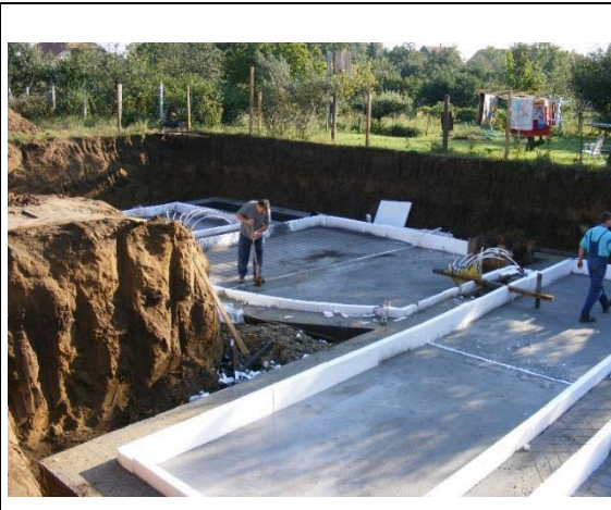
Figure 3b: Edge thermal insulation and covered tubing Photo T. Barkanyi
