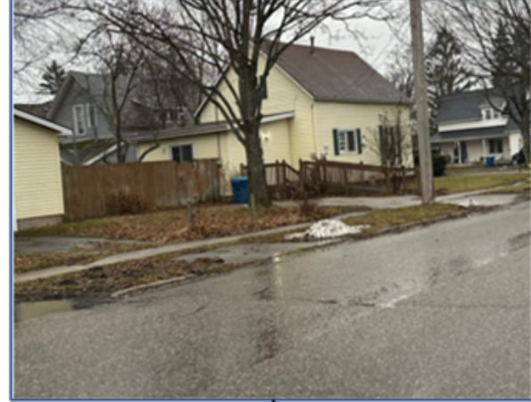
Gay St: Cracked and uneven sidewalk
