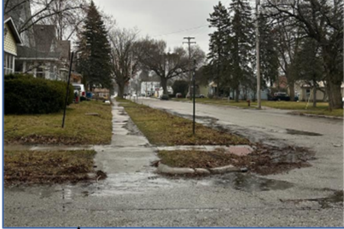
Gay St: Cracked and uneven sidewalk
