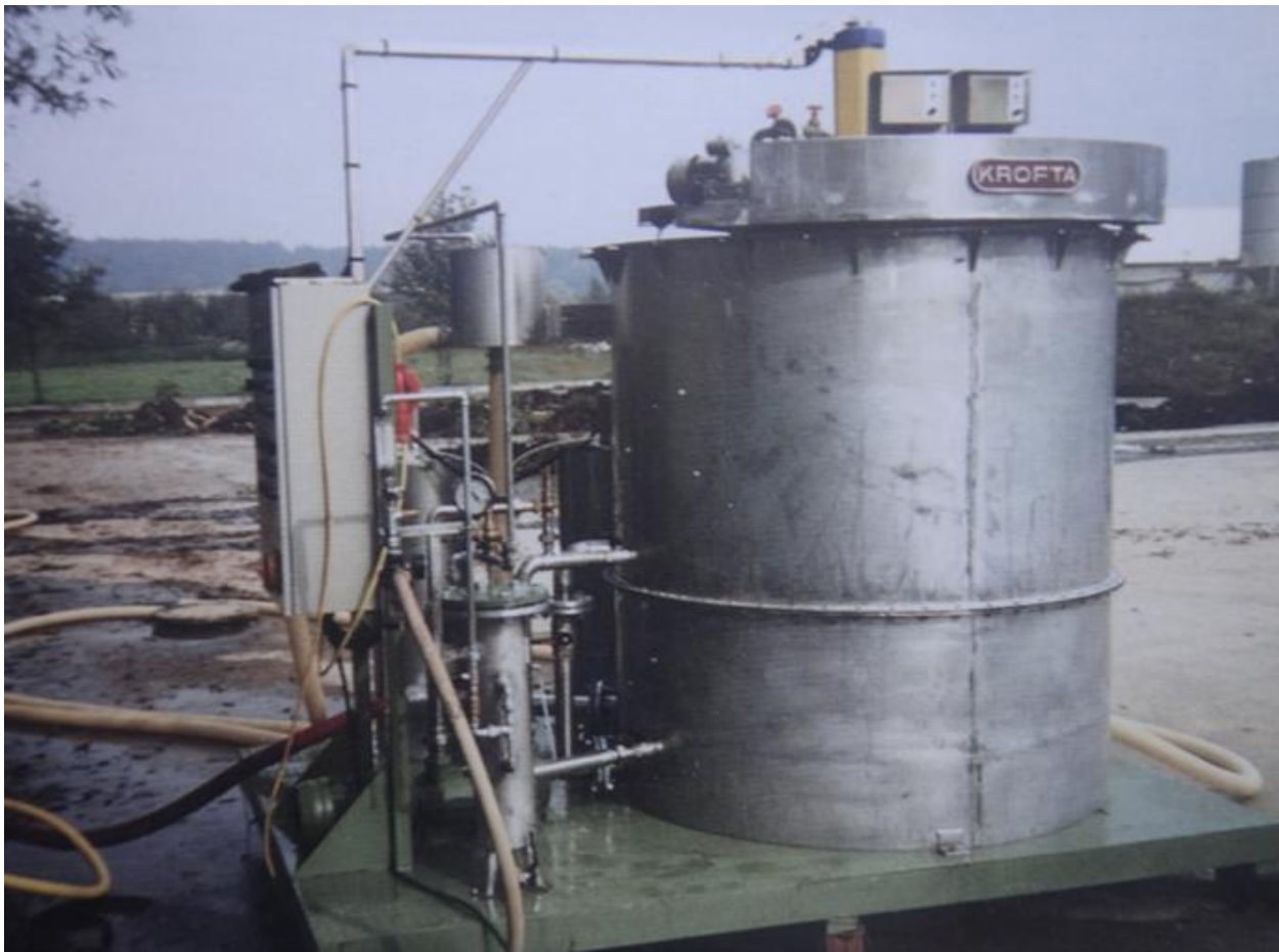
Figure 1. A complete Krofta Sandfloat DAFF water purification system in the field (Source: Lenox Institute of Water Technology)
