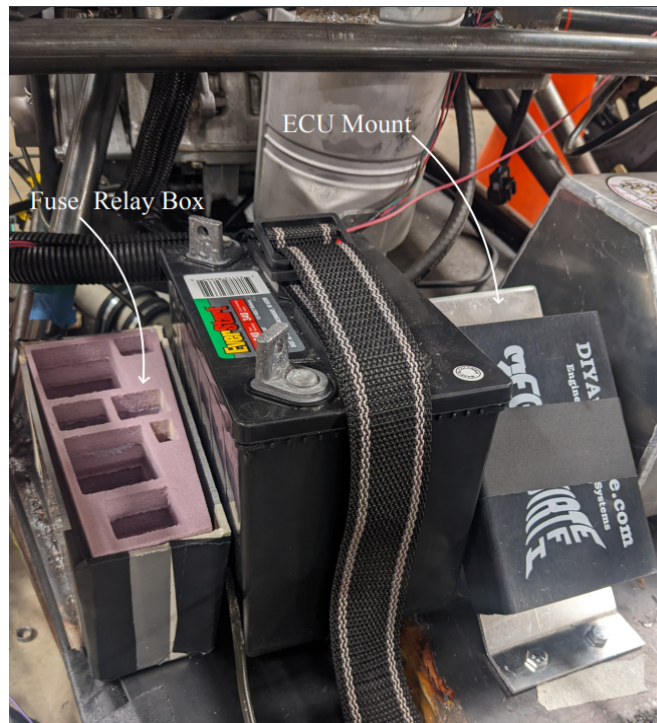
Figure 10: Other components that were added to improve the organization of the electrical system such as a reuse/relay box and mount for the ECU
