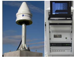
Figure 3.6: GESS antenna and cabinet.
