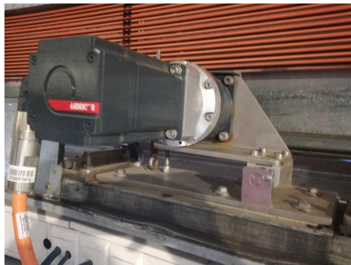
Fig. 2-46: Wood beam and motor for moving the dome
