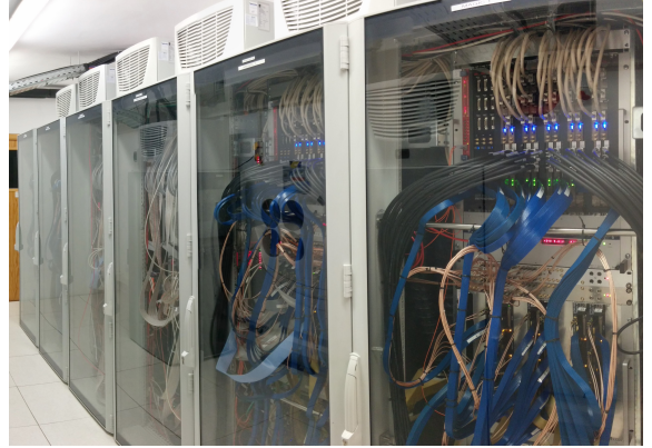
Figure 4: View of the electronics room of the MAGIC telescopes. The six closed racks can be seen. They are placed on a technical raised floor (20 cm height) allowing for better cable routing.
