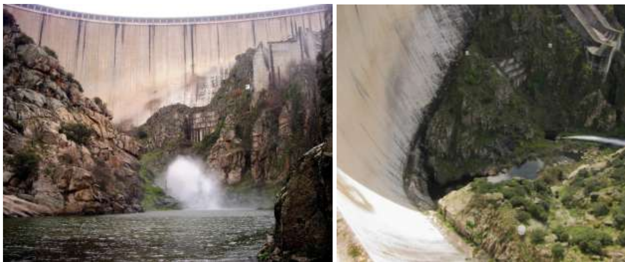
Fig. 5.4. Almendra dam shot from downstream (left) and upper view (right). The plume is the ‘ecological flow’ released through a Howell valve that never surpasses 500 liters per second. The water table in the forefront is contained in a little shock-absorber reservoir. Pictures taken by Ignacio Rodríguez.
