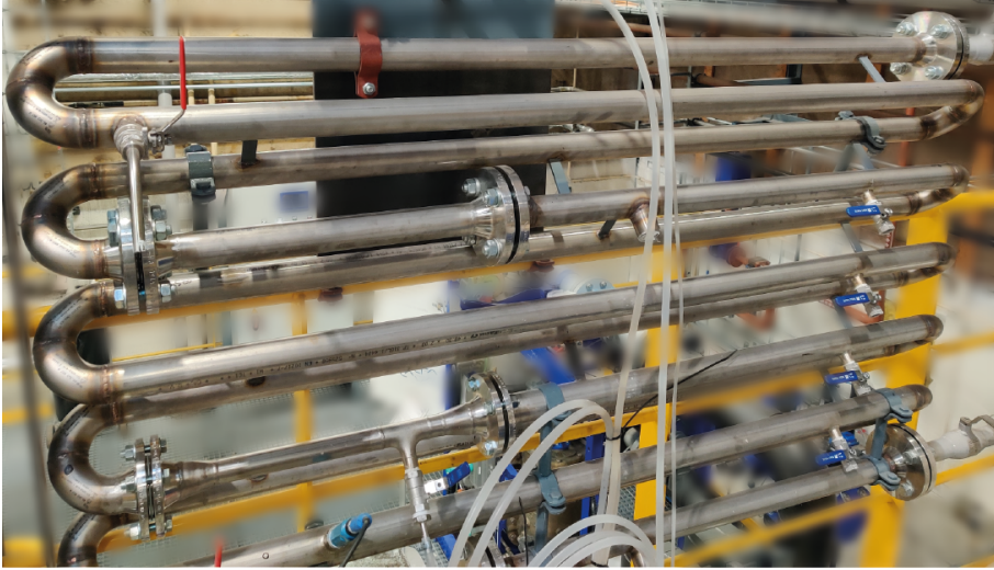
Fig. A.2: In-line pre-treatment static flocculator. The flocculator consists of a set of 180^\circ pipe bends and a metal coagulant is dosed at the inlet of the application and the dosing of the cationic polymer is performed after a total of 4 \times 180^\circ pipe bends. The particle size distribution is measured at the outlet of the static flocculator.
