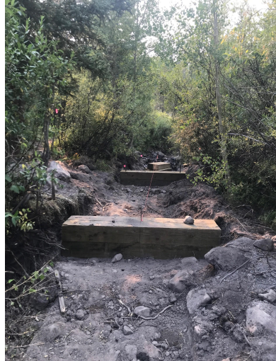
Figure 5. mud sills in ground
