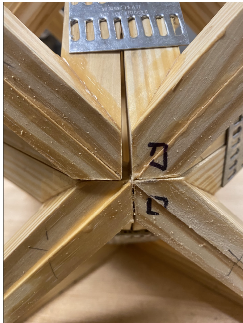
Figure 30: Gap between connections due to a fabrication error.
