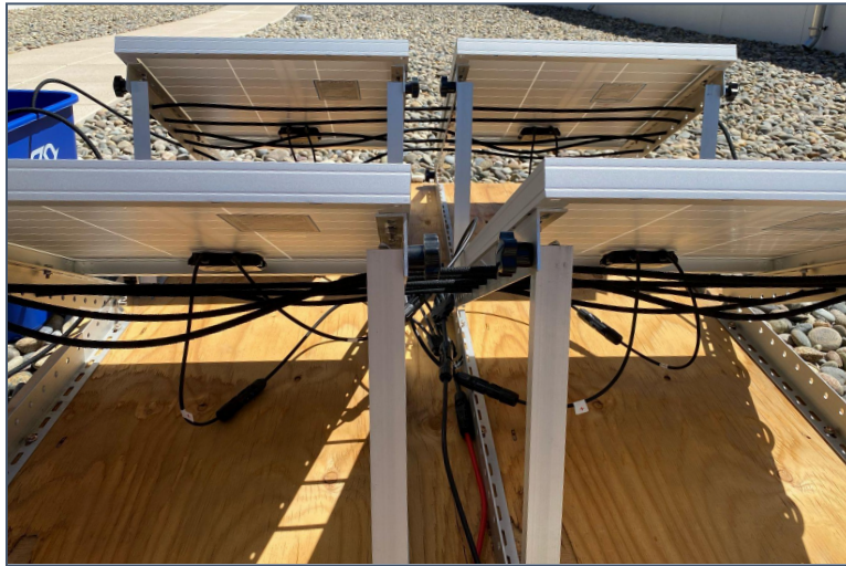
Figure 13: Back View of Cooling System
