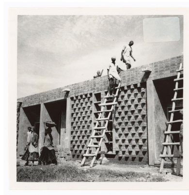
The titles for the photographs above are based on their respective inscriptions located on their verso. Jeet Malhotra or Pierre Jeanneret, View of houses for peons under construction, Sector 23, Chandigarh, India. ARCH402403, Pierre Jeanneret fonds, CCA. Gift of Jacqueline Jeanneret © CCA
