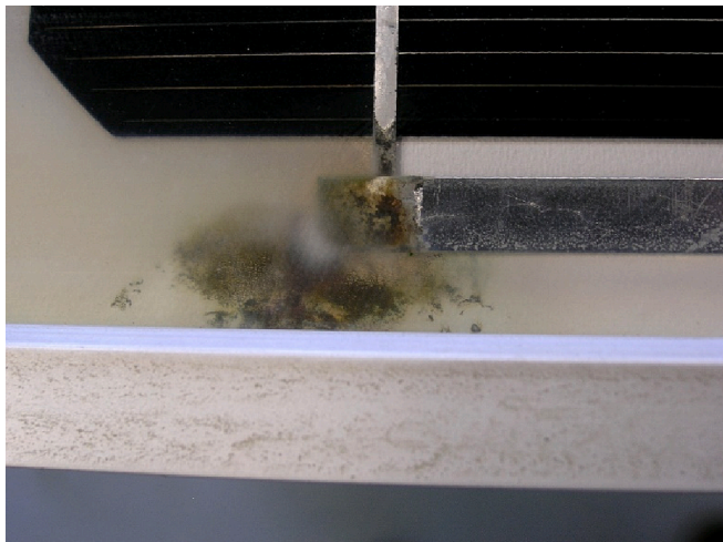
Fig. 3. Formation of a conductive channel between the electrode and the ground of the PV panel.
