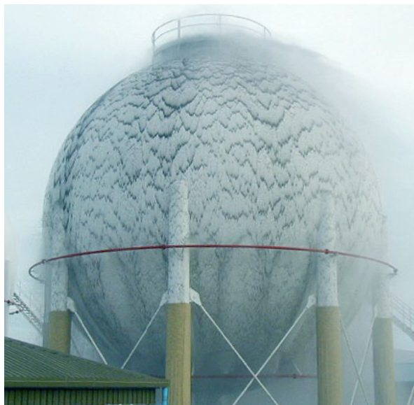
Figure 5.9 - Test of fire water system on spherical LPG storage tank (49)
