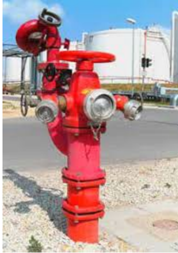
Figure 3.13 – Combination Unit (Hydrant/Fire Monitor) at a chemical plant
