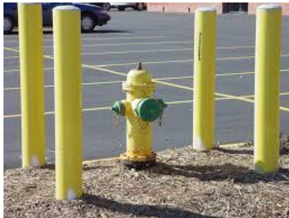
Figure 3.14 – Example of post guards protection a hydrant
