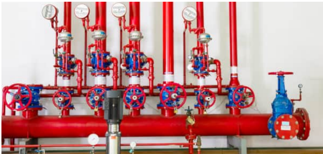
Figure 3.6 – Example of a manifold with several systems attached
