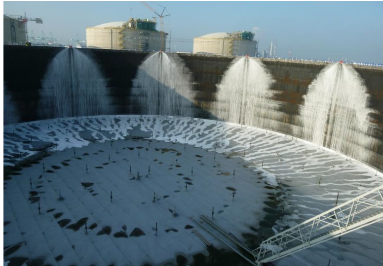
Figure 5.11 - Discharge outlets working in an Open top Floating Roof Tank (52)
