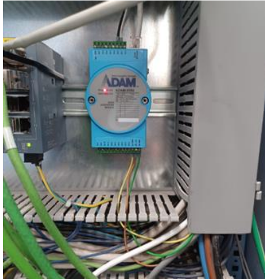
Figure 4.5 - I/O module installed in the equipment's electrical panel.
