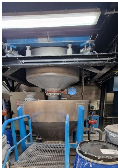
Figure 22 - Fixed tank for filling on the ME-32
