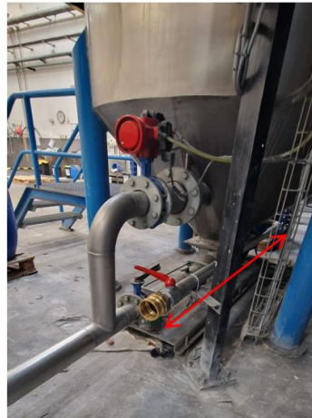
Figure 32 - Fixed tank pipe extension for purging in the ME-32 machine
