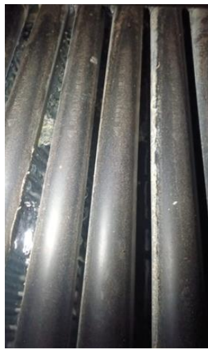
Figure 28- Interior pipes of the ice bank before using biocide.
