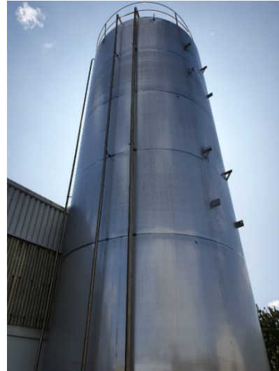
(b) Storage tank
