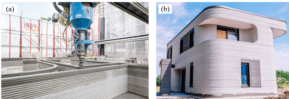
Figure 2.5: Germany's first concrete 3D printed residential building (a) during construction and (b) when completion (Ozdemir, 2021)
