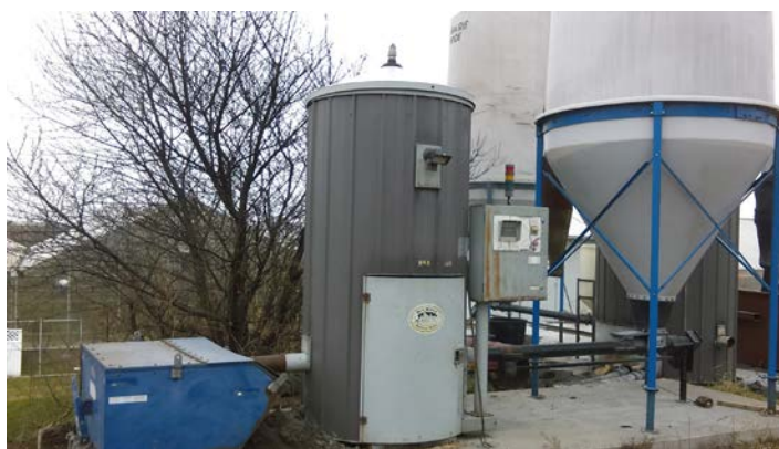
Image 5.2 Pork and Plants boiler
