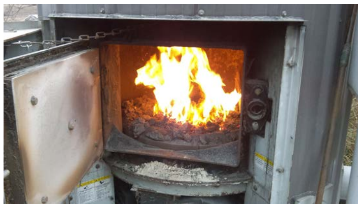
Image 5.3 Pork and Plants boiler
