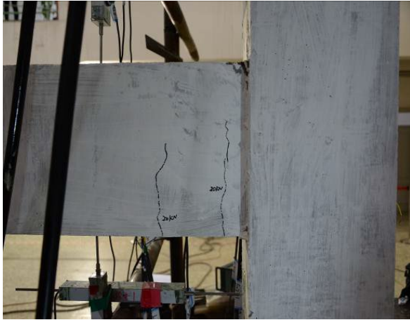
(a) First observed crack in the beam
