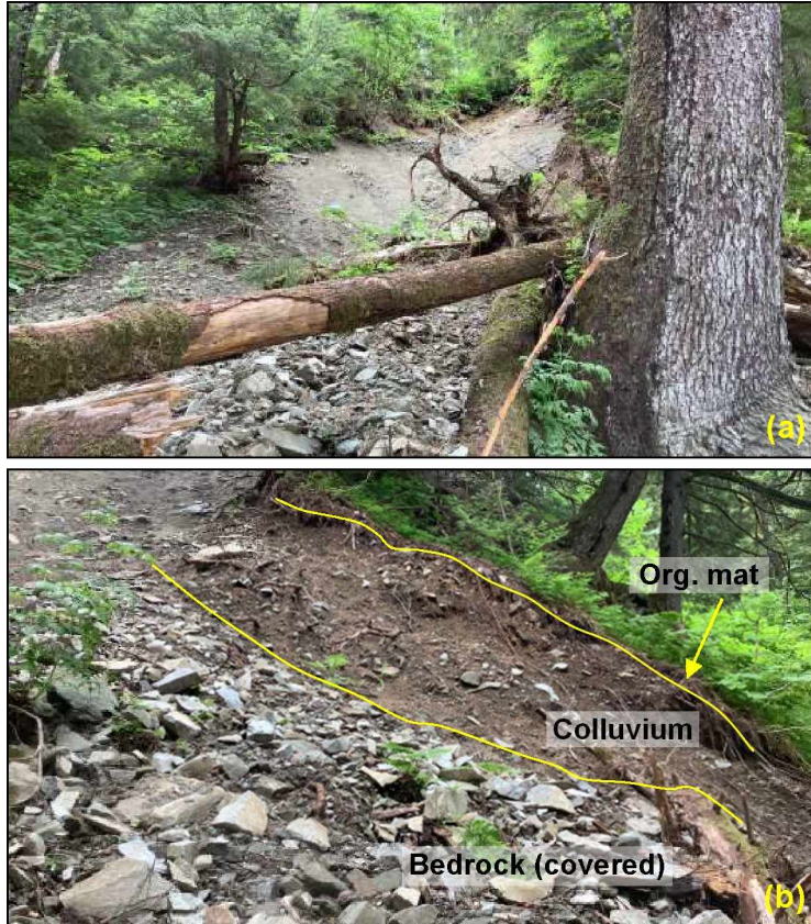
Figure 30. Photographs of FEMA DOT#19 (June 2021): (a) view of head scarp from road level; (b) left flank showing approximately 2 m of brown colluvial material; the diorite bedrock exposed near the head scarp was mostly covered by debris at this location.
