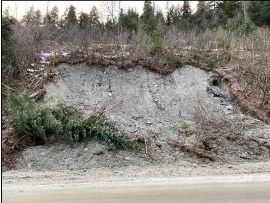
Figure 88. View of the failure at FEMA DOT#46 from Lutak Road in December 2020 (photograph courtesy of ADOT&PF).
