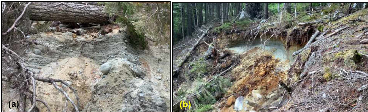
Figure 16. Photographs of the VP sand flow slide (June 2021) showing: (a) stratigraphy exposed in the left flank at the slope base, showing alternating fine and coarse sand layers with interspersed gravel and cobbles; (b) the head scarp, as seen from the left flank, with iron-cemented sand both intact beneath the organic mat and loose on the slope.
