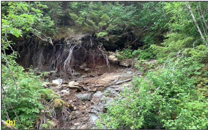
Figure 77. Views of the affected area at FEMA DOT#41: (a) slope in December 2020 (photograph courtesy of ADOT&PF); (b) head scarp area (June 2021).
