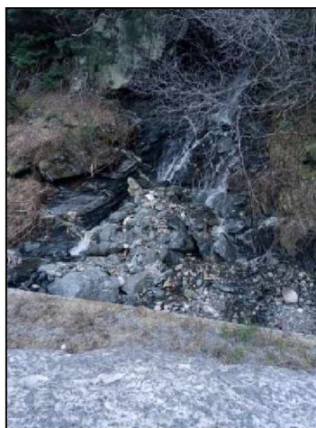
Figure 122. View of debris in the channel at FEMA DOT#63 in December 2020 (photograph courtesy of ADOT&PF).
