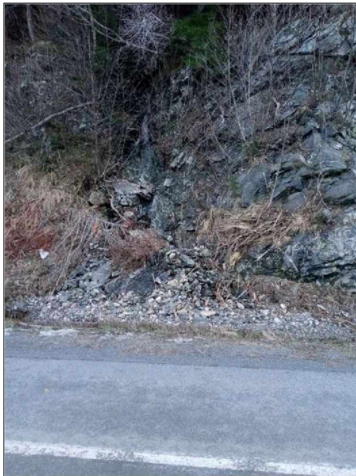
Figure 128. View of debris in the ditch at FEMA DOT#62 in December 2020 (photograph courtesy of ADOT&PF).
