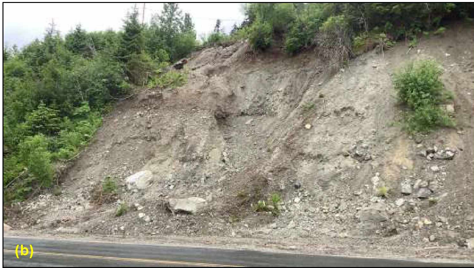
Figure 90. Views of the FEMA DOT#47 slide area in: (a) December 2020, following clean-up efforts (photograph courtesy of ADOT&PF); and (b) June 2021.
