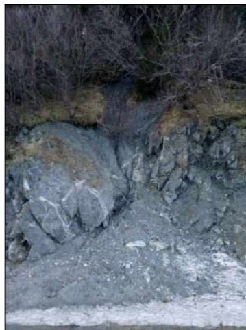
Figure 124. View of debris in the ditch at FEMA DOT#58 in December 2020 (photograph courtesy of ADOT&PF).
