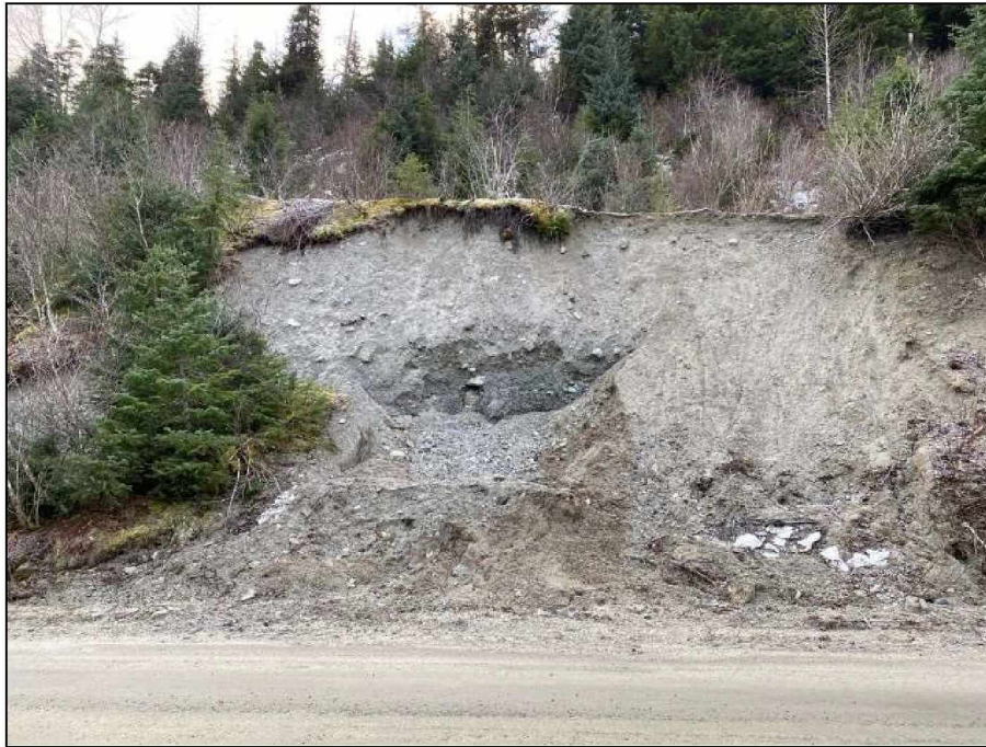
Figure 86. View of the failure at FEMA DOT#45 from Lutak Road in December 2020 (photograph courtesy of ADOT&PF).
