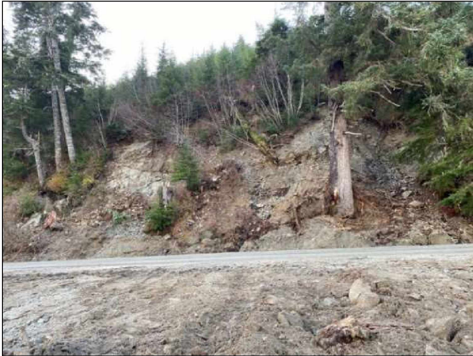
Figure 40. View of slope failure at FEMA DOT#24 from Lutak Road in December 2020, post clean-up (photograph courtesy of ADOT&PF).
