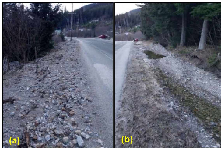
Figure 113. Views of FEMA DOT#65 in December 2020, illustrating (a) debris that was pushed off the road and (b) debris that was caught in the ditch (photographs courtesy of ADOT&PF).
