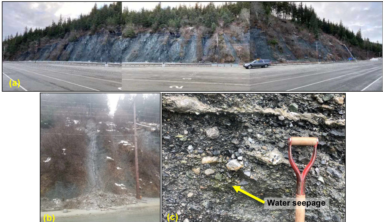
Figure 95. Photographs of the slope adjacent to the ferry terminal (FEMA DOT#49): (a) the entire extent of the slope across Lutak Road from the ferry terminal, post cleanup (December 2020; photograph courtesy of ADOT&PF); (b) an individual debris flow in December 2020 (photograph courtesy of ADOT&PF); (c) view in June 2022 of soil at sample location 22-07 and 22-08, demonstrating ongoing water seepage (note the algae growth in the left side of the image).
