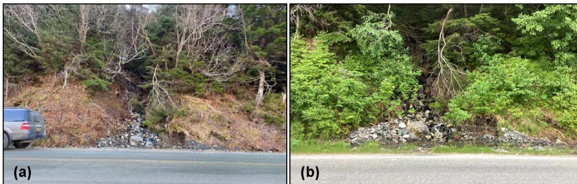
Figure 44. Photographs of FEMA DOT#26 channel in (a) December 2020 (photograph courtesy of ADOT&PF) and (b) June 2021.
