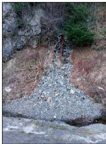
Figure 126. View of debris in the channel and ditch at FEMA DOT#61 in December 2020 (photograph courtesy of ADOT&PF).
