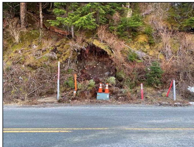
Figure 69. View of the failure at FEMA DOT#37 from Lutak Road (photograph courtesy of ADOT&PF).
