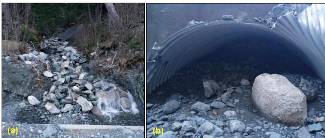
Figure 118. Photographs of the Johnson Creek location in December 2020: (a) the channel from Lutak Road; and (b) culvert filled by debris (photographs courtesy of ADOT&PF).
