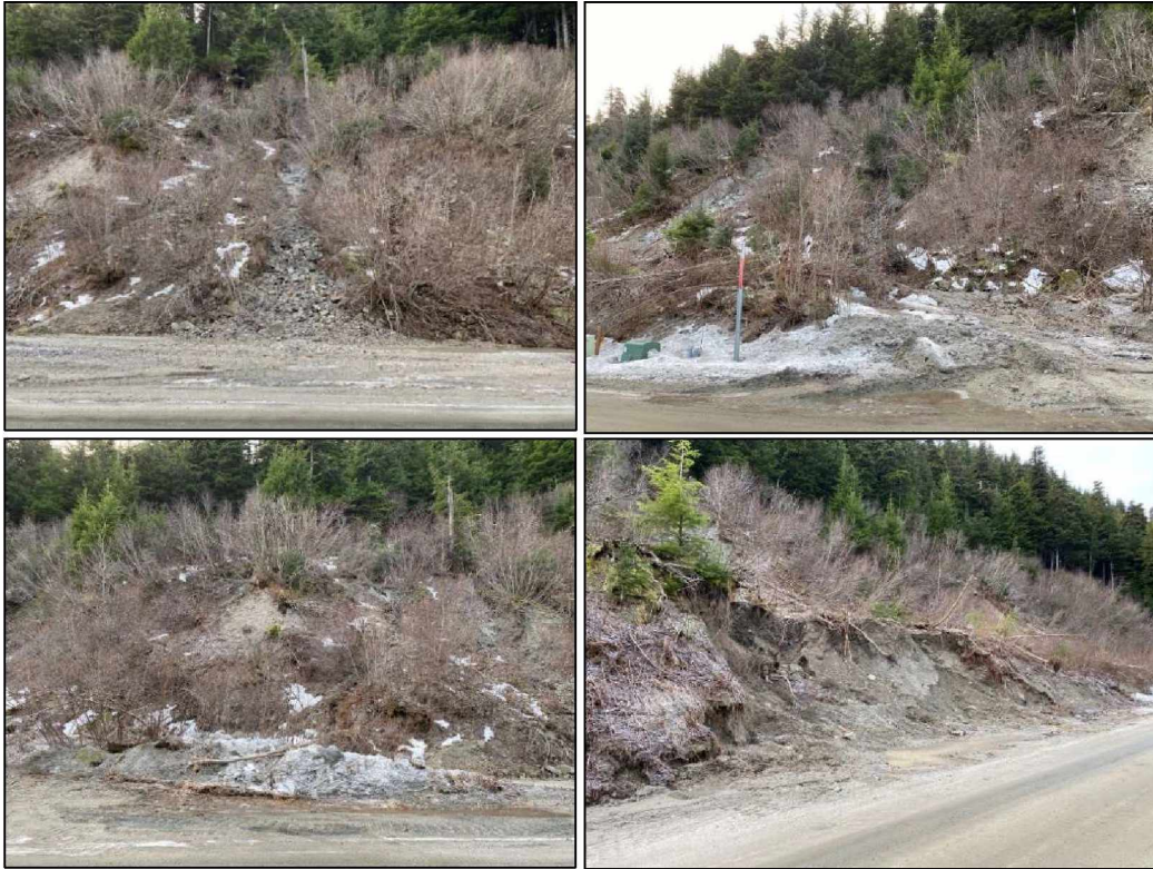
Figure 84. Collection of photographs of the FEMA DOT#44 landslide area in December 2020, showing evidence of both debris slides and debris flows (photographs courtesy of ADOT&PF).
