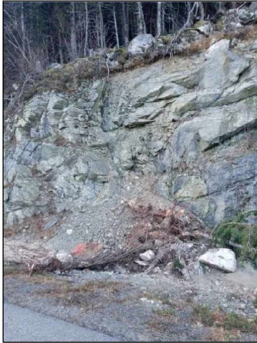
Figure 130. View of the FEMA DOT#59 slope with debris at its base in December 2020 (photograph courtesy of ADOT&PF).
