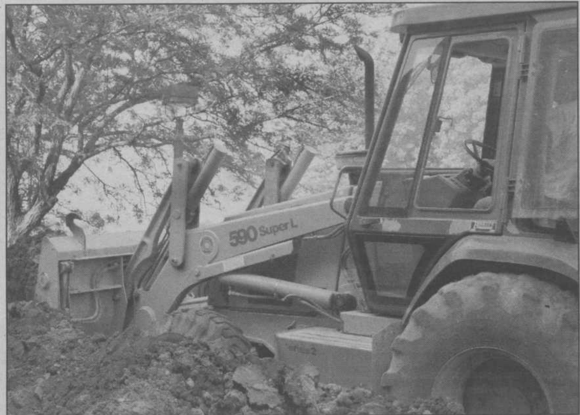
Kevin Butler, of Tolono, works Monday morning on the west side of the C-Wing on the roof drainage project. Other work on campus is being done on sidewalks.
