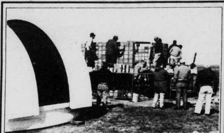
Workers are finishing work on the observatory, local in rural Champaign. The observatory will be maintained by the Champaign-Urbana Astronomical Society.
