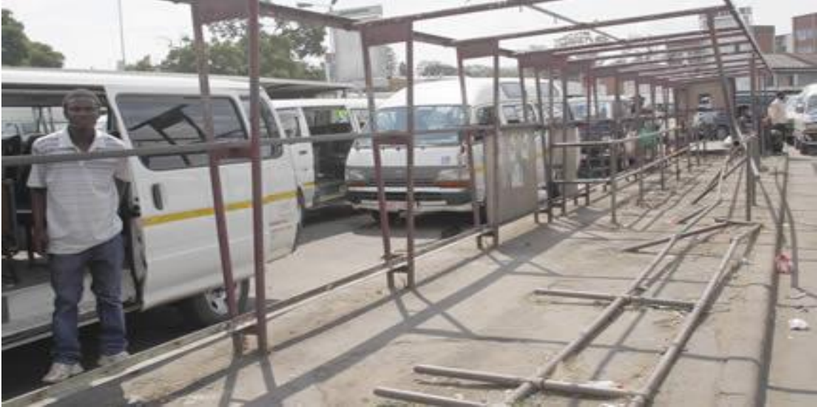
Plate 6-4. Dilapidated public transport termini shelters. Source: Author
